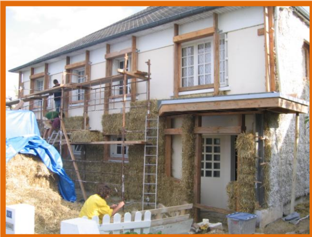
This house in France is being retrofitted using strawbales. Using the same approach here could lead to new local businesses, skills and retraining. Photo: Yannick Molin.
